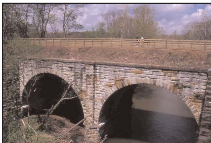
The Stone Viaduct just west of Norwalk is NOW OPEN to trail users. New safety fencing complements the structure. See page 2 for details.
