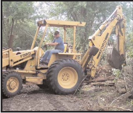
As Mallory maneuvers his backhoe through the jungle, one can see the future trail surface take shape.
