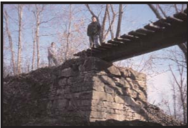
Kate Mantey and Stan Bernhardt inspect the stone culvert near Medusa Road last November.
