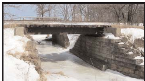
Similar to the recently completed Seymour Creek Bridge, only a little higher, Meggison Creek's Bridge will soon link east and west.
