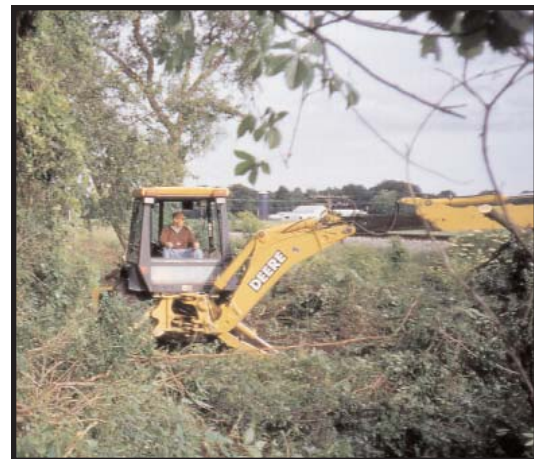
This view looks west near Sand Hill Road where work will soon begin to really push the trail west from Monroeville. Pictured is volunteer “trail blazer” Jim Wasiniak clearing the way.
