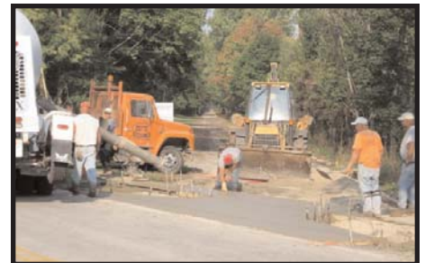
Oglesby Construction poured aprons at Rt 547 along with new sidewalks. A smooth transition, along with a safe road crossing, complete this shady stretch of trail. West of 547, the trail runs through the trees for 1.6 miles to Williams Road.
