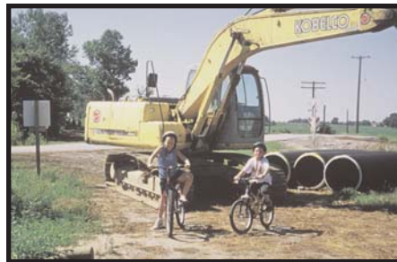
Haynes Construction graded the trail, cleared ditches, installed drainage pipe, and spread limestone between Jackson Street and Sand Hill Road. The equipment, here at Williams Road, is now gone, and kids of all ages are ready to ride into new territory.
