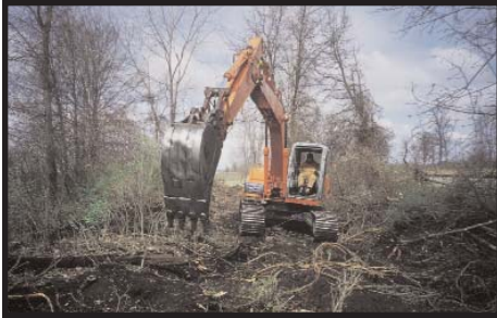
Jim Wasiniak's volunteer efforts led the way as the trail pushed west from Monroeville. His generous in-kind service contributions were of utmost importance to FRTTI in meeting their match to ODNR. The excavator used for the project was provided by Mark Schaffer.
